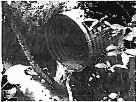
Photo 1. This culvert located on lower Bigelow Creek is impassable to fish moving upstream from Seymour Creek.
