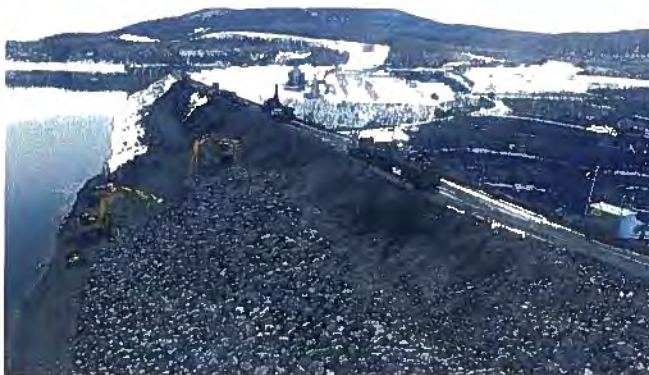
Approximately 135,000 cubic metres of rip-rap and bedding materials will be placed on the upstream face of the dam.
