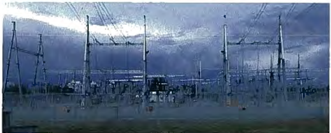
Shell Groundbirch Substation near Chetwynd.
