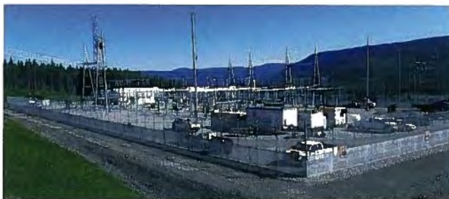
Meikle Terminal is a new substation that connects the wind farm with our electrical transmission system.
