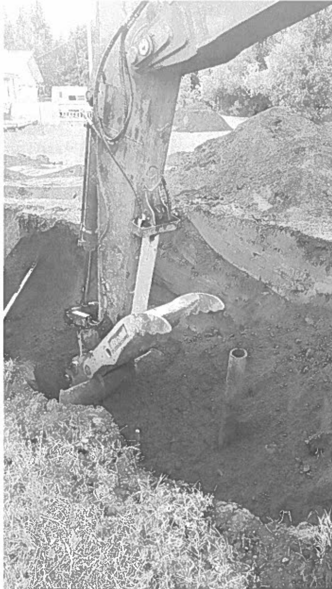
FIGURE 2 – BROKEN WATERMAIN ON 6 TH AVENUE
